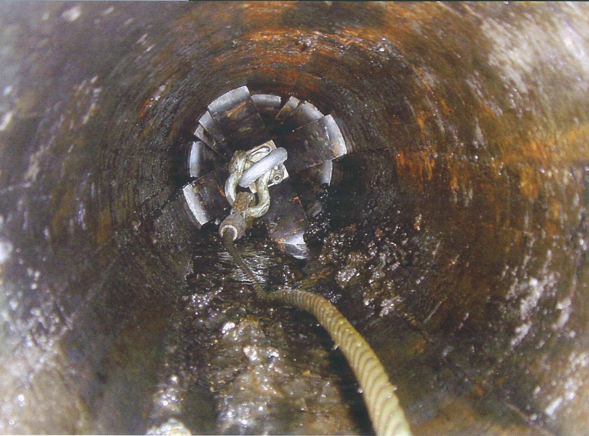
The drag scraper is pulled through the pipe to clean the walls before epoxy lining. Note the chatter marks on the walls. (Photos courtesy of Triton Lining Technologies)
