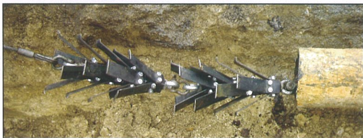
A winch system pulls pairs of clamped custom-made drag scrapers into the pipe to clean it. In Marion, Ind., the encrustation and tuberculation were so hard that it took 12 or more pulls to clean each section.
