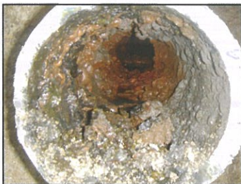
The tuberculation in the 4-inch cast-iron water main reduced flows by 50 percent.
